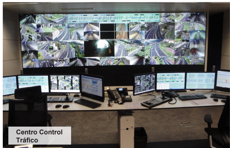
Sala de Control Build Management System
